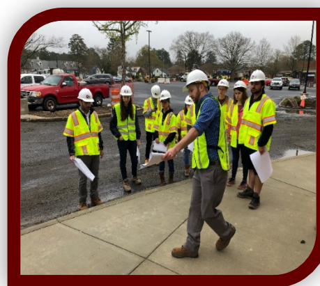
AES' Graham Corson describes an ADA-compliant sidewalk at the Midtown Row project in Williamsburg
